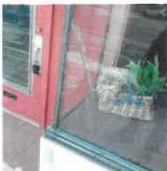
Figure 1 Front Window – Broken Glass
