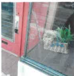
Figure 1 Front Window – Broken Glass
