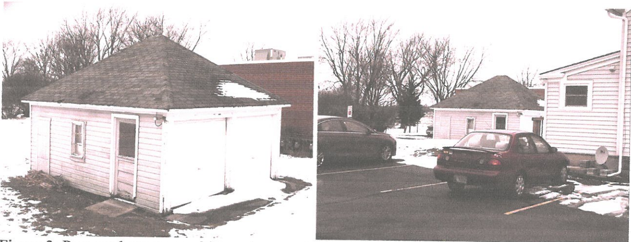
Figure 3: Proposed garage roof for replacement and visibility of garage roof from public right of way.
