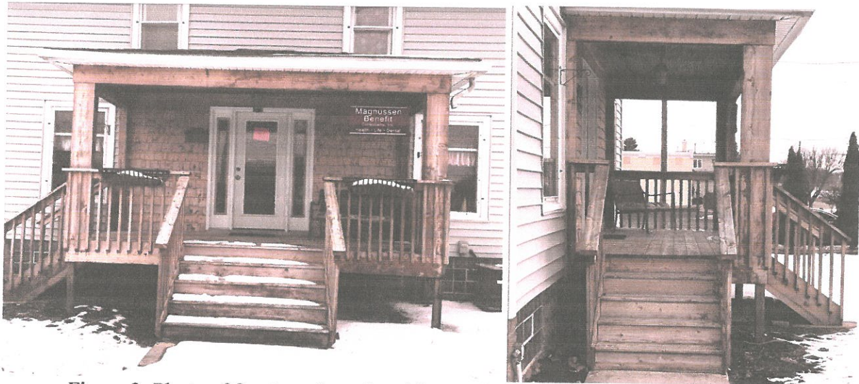
Figure 3: Photo of front porch, cedar siding and stairs for proposed painting work.
