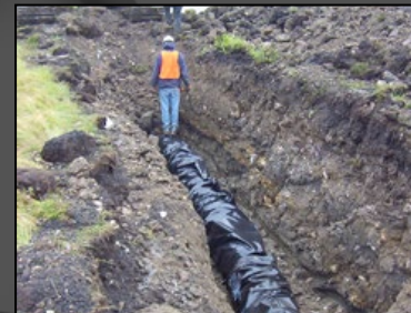
Water Distribution & Storage
