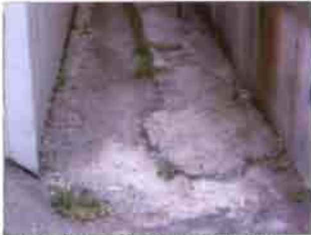
The sidewalk between Block Brothers and the garage is disintegrated
