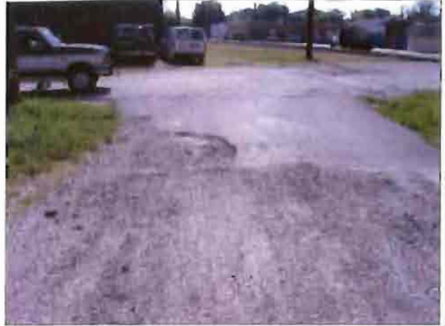
The un-platted alley way south of Mill Street is deteriorated.
