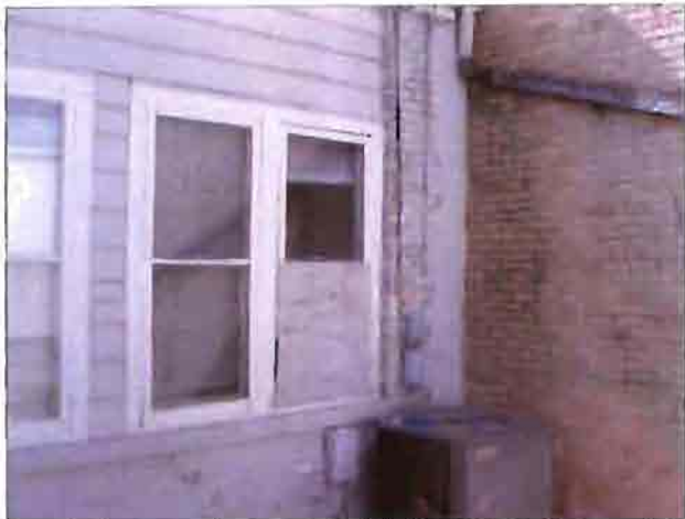
Boarded up rear window at the Medical Clinic. Note: paint peeling from brick.
