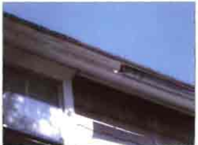
Deteriorated and missing sections of gutter on the single-family fronting Washington St.
