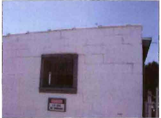
The secondary structure on the propane storage facility has rotting window framing and step cracking in the masonry block walls.
