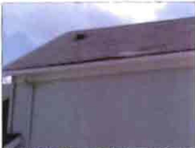
The roof on the bank next to the SBC building is in need of repair.
