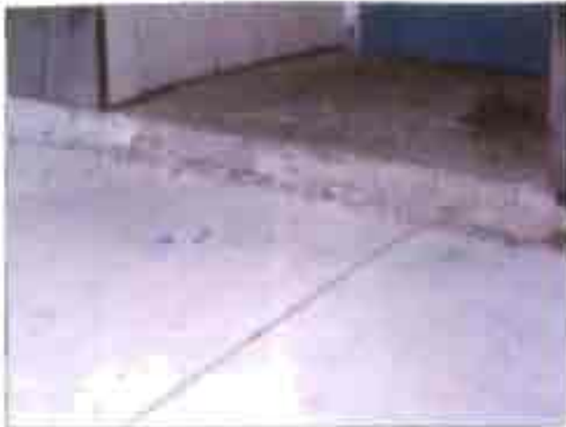
Concrete slab at Lydo's Pizza entry is cracked and crumbling
