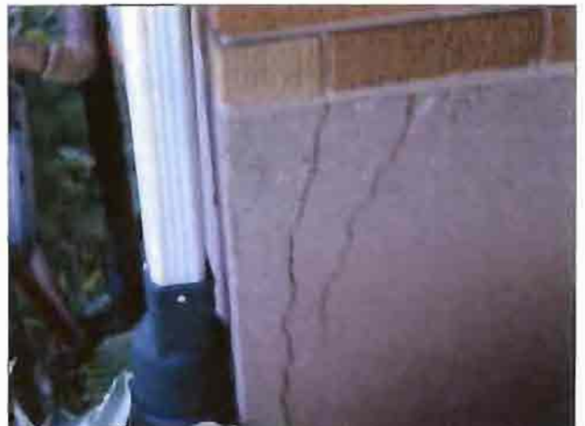
The foundation is cracking on this single-family fronting State Street.
