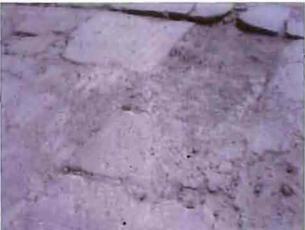
Dilapidated parking lot on the west side of State Street.
