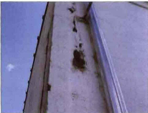
Block wall at rear of the Country Lanes building where the old downspout has been removed has large holes.
