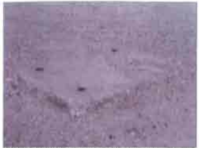
Old sign base located in the middle of the entrance to the SBC building off of the alley. Note crumbling pavement
