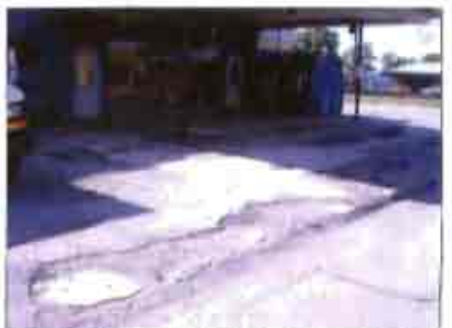
The parking lot in front of the NAPA store is riddled with pot holes, cracked and crumbling
