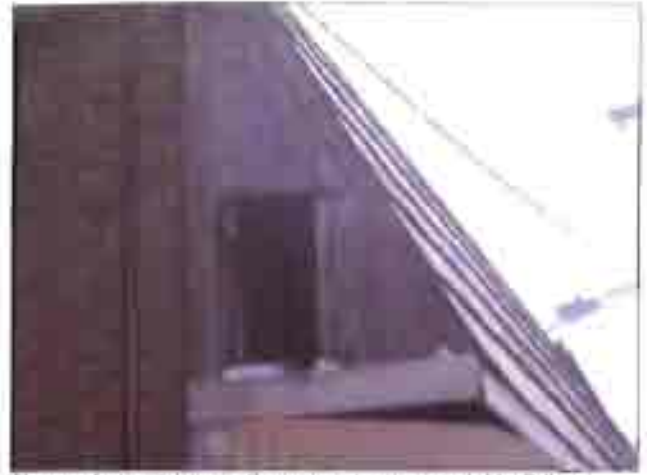
The roof structure on the vacant commercial building behind NAPA is rotting and the soffit is pulling away from the roof overhang.
