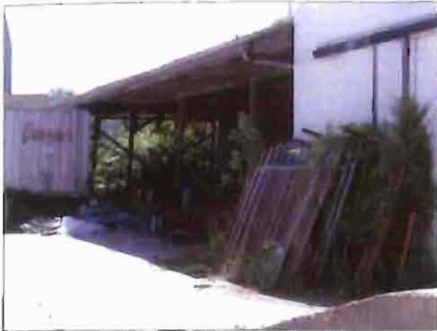
The gutters on the canopy in the rear of the Seagren's parcel is peeling away from the structure. Note: weeds overgrowing old fence sections.
