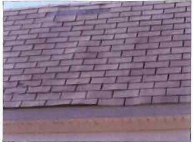
The roof on the Fitness Center is missing sections of shingles and is coming loose.
