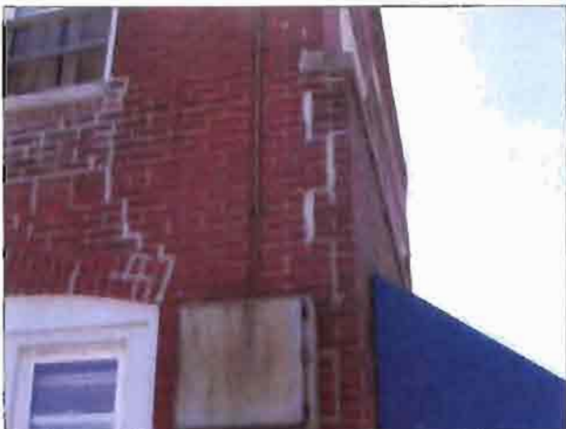
Patched step cracking on the side of the Hampshire Township building.
