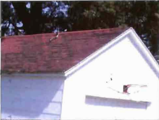
The roof on the garage in the rear of the single-family house at the corner of Mill and East is severely deteriorated.
