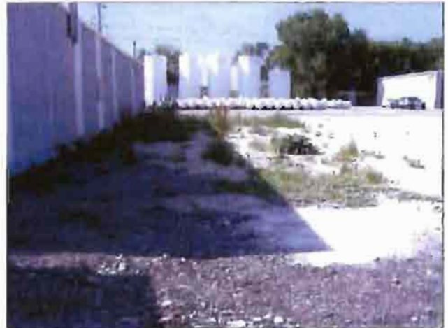
Deteriorated parking lot, overgrowing with weeds at one of the industrial properties located on Mill Street.
