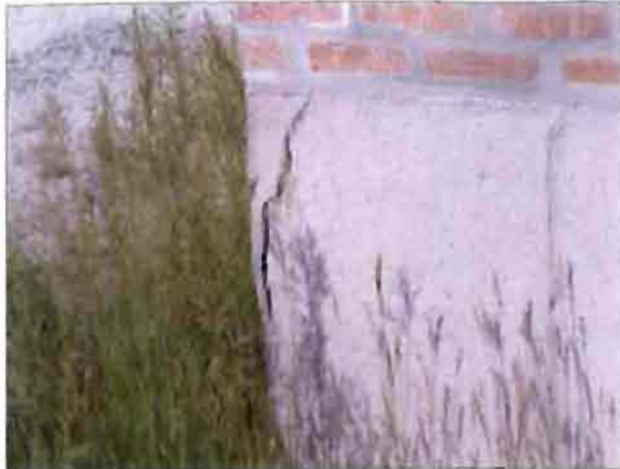
The foundation on the recently renovated Office Condos fronting Mills Street is cracking.
