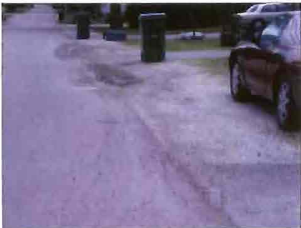
Typical pavement shoulder deterioration and evidence of ponding water.
