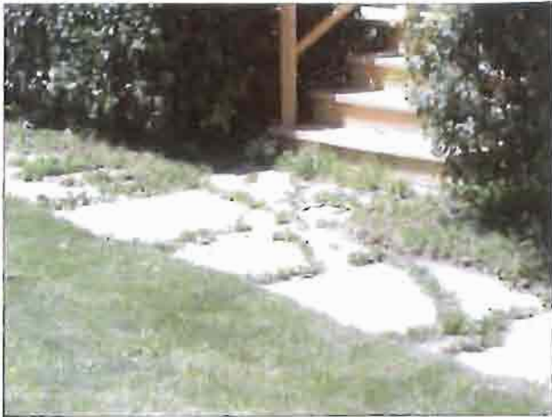
The sidewalks along Keyes Avenue are severely deteriorated.
