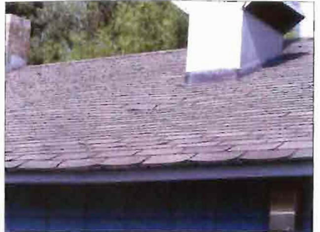
Deteriorated roofing material on the barber shop fronting Washington St. Note: sagging in roofing structure.
