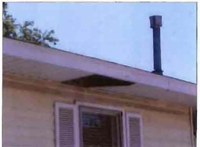
Missing sections of soffit on single-family south of Keyes Avenue.
