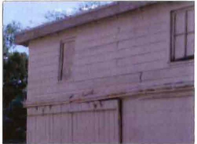
The wood siding and fascia boards on the Fitness Center are deteriorated.
