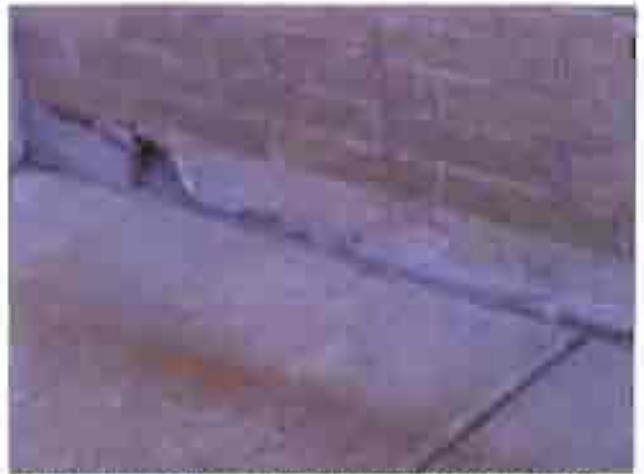
Foundation cracking and crumbling on the north side of the American Bank Building.
