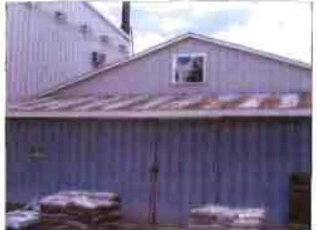
The roof on the garage north of Block Brothers is rusting.
