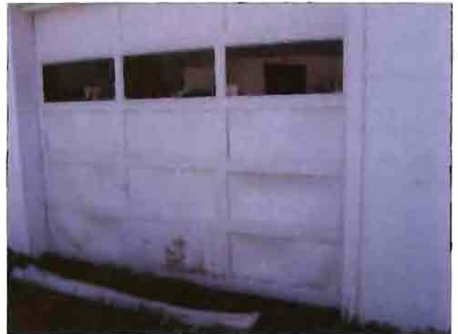
The garage door is rotting and warped on the previously mentioned industrial property.
