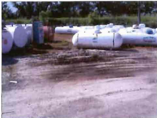
Deteriorated parking lot on the propane storage facility
