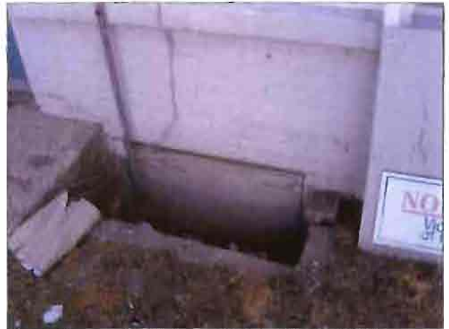
Cracked concrete window well at the Medical Clinic. Boarded window subject to water damage .
