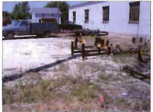
The parking lot at the corner of State Street and Keyes Avenue is deteriorated.
