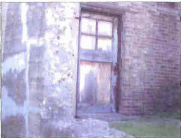
Rotted door on the industrial building south of Keyes Avenue. Note: patched concrete wall.
