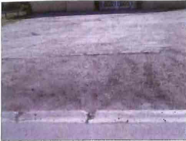
The parking lot in front of the Fitness Center is severely deteriorated.
