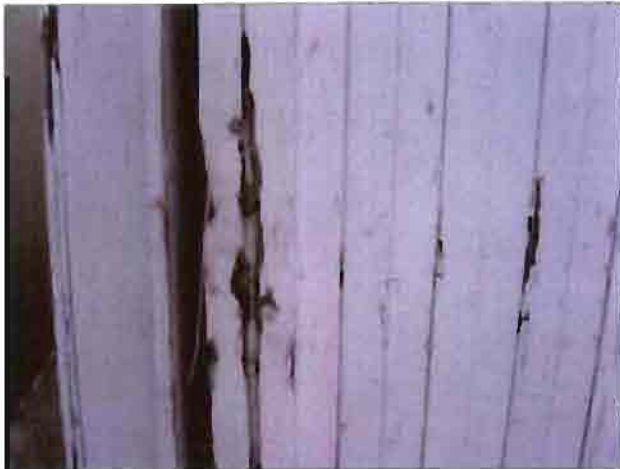
The wood siding on the previously mention industrial property is rotting.
