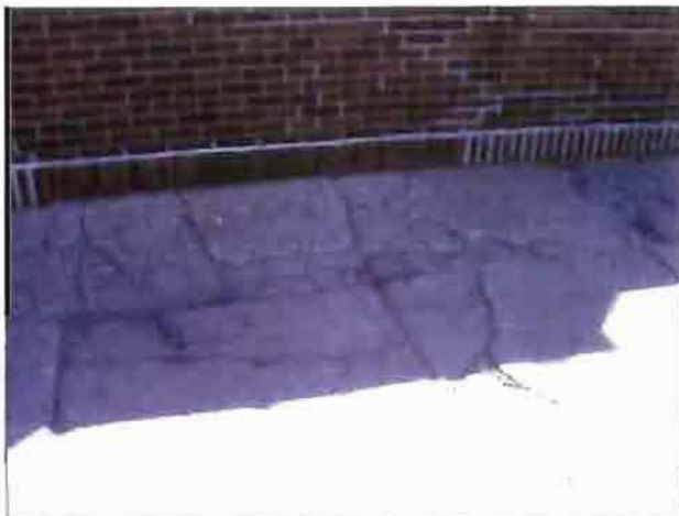
The sidewalk along State Street is deteriorated.
