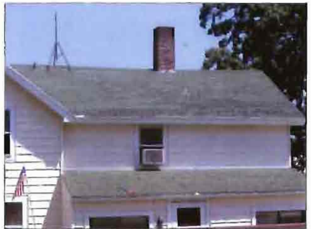
The roof on this single-family south of Keyes Avenue is deteriorated. Note: damage to shingles.
