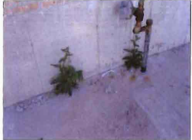
Weeds growing between the foundation and the sidewalk of the Office Condos on Mill Street.
