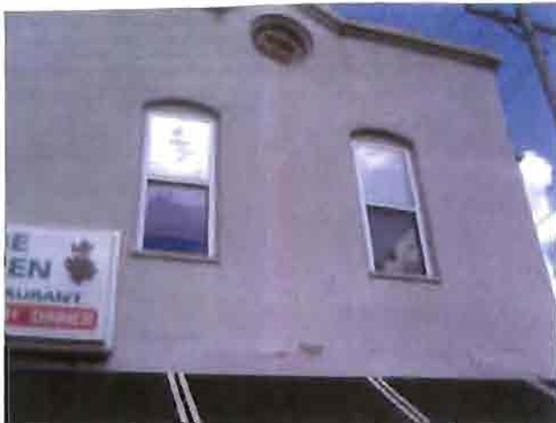
Stucco veneer on the front of the Rose Garden is cracking and separating from masonry surface indicating moisture problems..
