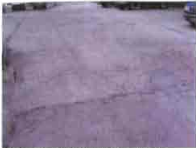
Deteriorated parking lot behind the SBC building.
