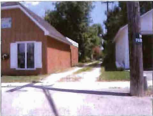
Typical deteriorated alley with grass growing.
