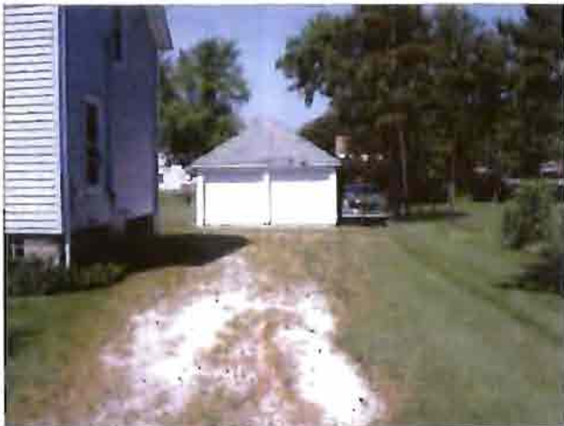
Deteriorated driveway leading to the garage in the rear of the single-family fronting State Street.
