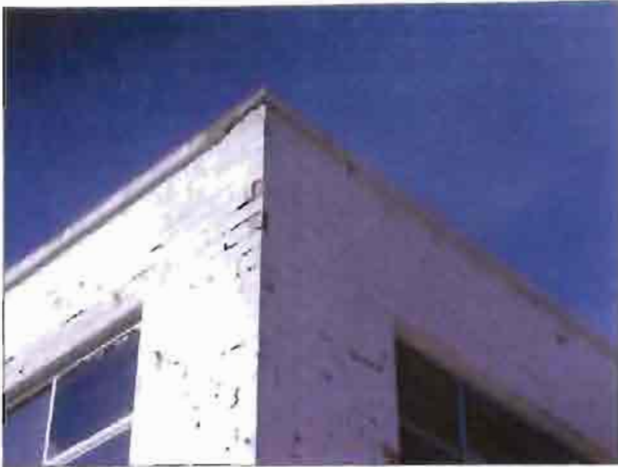
The paint on the bricks on industrial building on Mill St. is spalling indicative of moisture build up in the brick.
