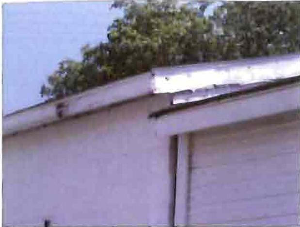
The soffit and fascia is rotting on the industrial building east of Center Street. Also, missing gutter.
