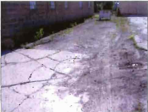
Severely deteriorated pavement on Animal Hospital parking lot.
