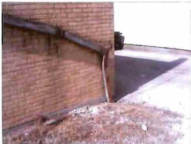
Rusted gutter and downspouts on the Medical Clinic.
