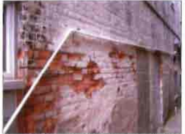
The brick on the south side of Village Hall is disintegrating
