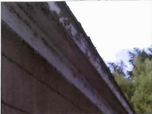
Paint peeling from the soffit and fascia on the barber shop fronting Washington St.
