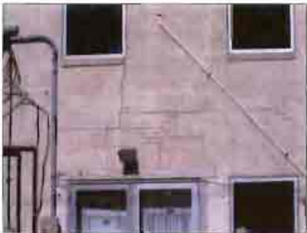
The rear of the Drey Miller Meat Building. Some effort has been made to re-mortar step crack in brick wall.
