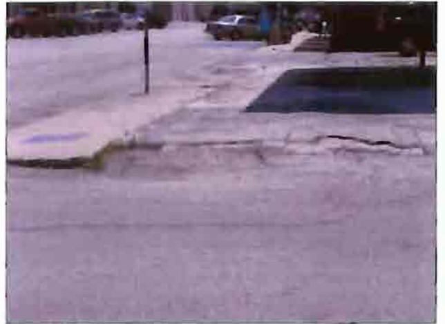
Many of the aprons throughout the Area are cracked and crumbling.
