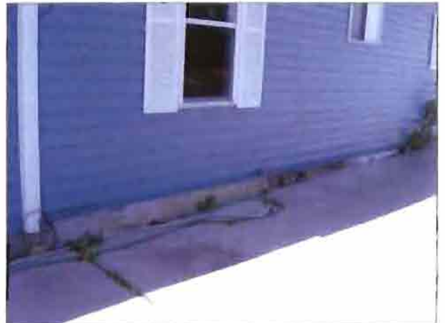
Cracking and crumbling foundation on the single-family dwelling at the corner of Mill and State Street.
