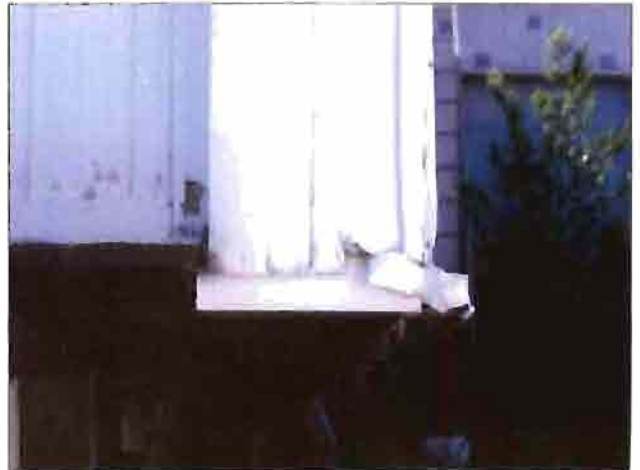
The wood siding on the Pets at Peace Crematory is rotting.
