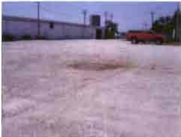
The parking lot in front of this industrial building is deteriorated and has large pot holes.
