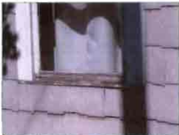
Deteriorated window frame and sill on the single-family home fronting Washington St.
