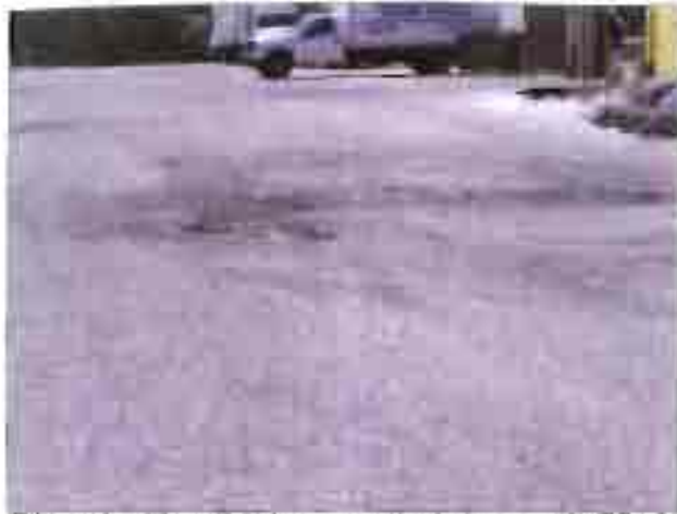
The parking lot on this industrial parcel south of Industrial Drive is cracking and crumbling.
