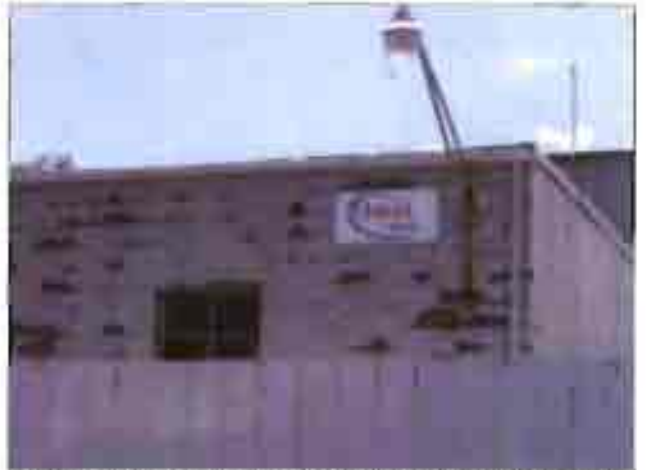
Paint separating from the front of the concrete block wall on front of the Omni-tech building is indicative of moisture damage.
