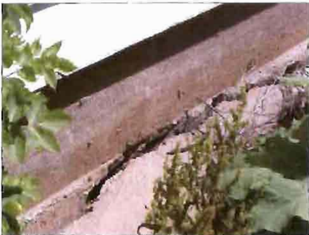
The foundation on the middle building on the Seagren's parcel is cracking.
