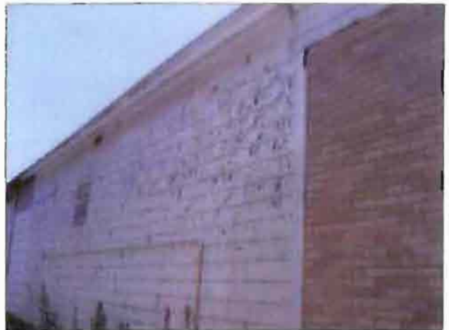
The paint is peeling off of the middle building on the Seagren's parcel.
