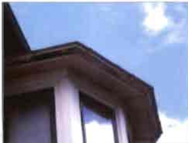
The soffit and fascia on Sue's Beauty is rotting
