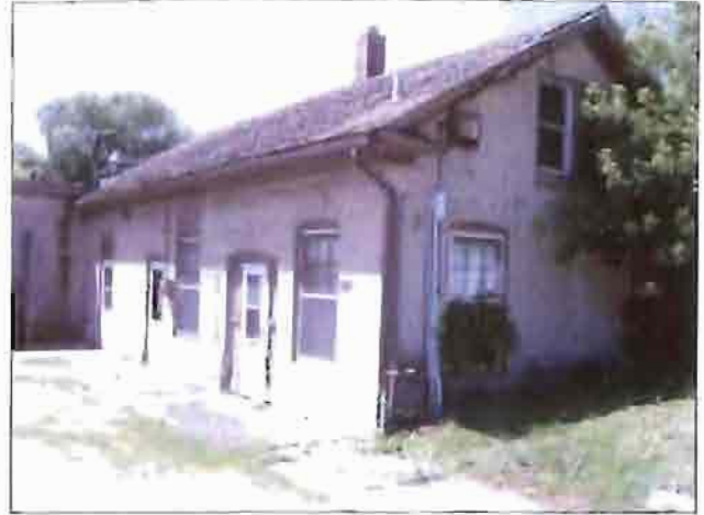
The roof on this industrial building south of Keyes Avenue is deteriorated. Note: damaged shingles.
