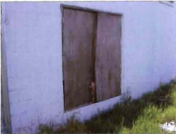
The door in the rear of the Country Lanes is warped and needing replacement.
