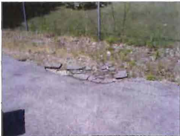
Sections of Keyes Avenue have inadequate shoulder and pavement is breaking apart (typical along street).
