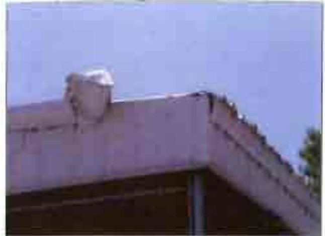
Damaged fascia on industrial building south of Industrial Drive.
