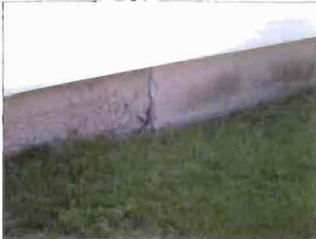
The foundation is crumbling on this single-family south of Keyes Avenue.
