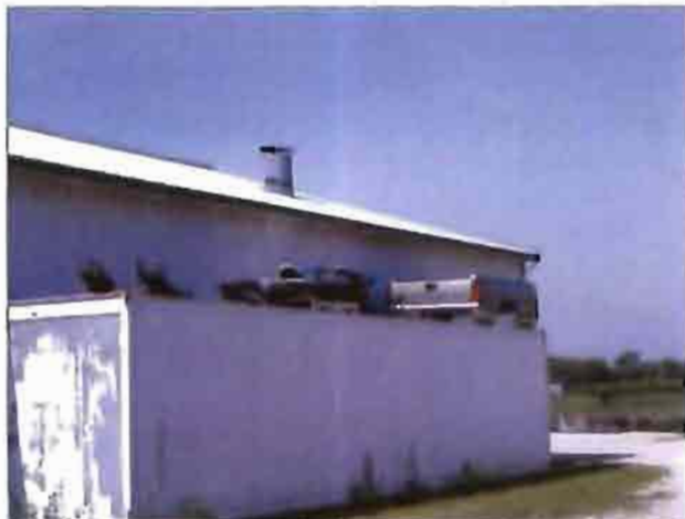
Salvaged vehicle parts being stored on the roof of a trailer in the back of the School Bus Maintenance Building.
