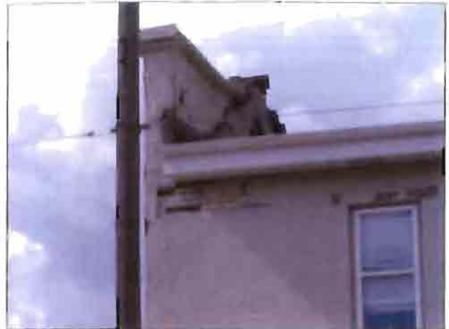
The south side of the Rose Garden. Dilapidated front parapet wall has since been removed.
