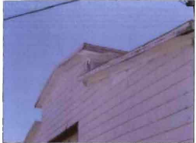
The paint on the soffit and fascia is peeling and the boards are starting to show water damage.
