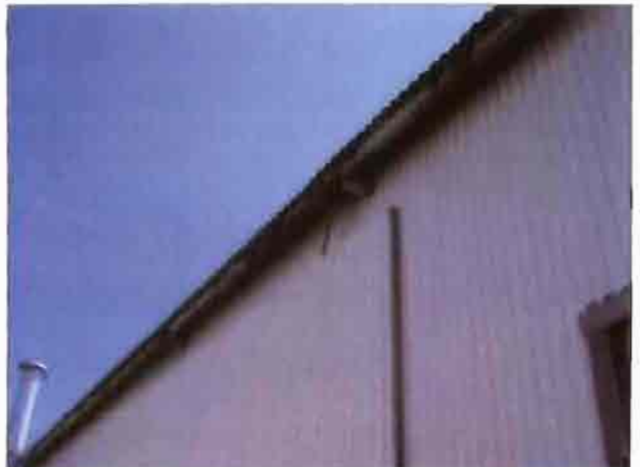
Rotting fascia is falling off of the industrial building north of Center Street.
