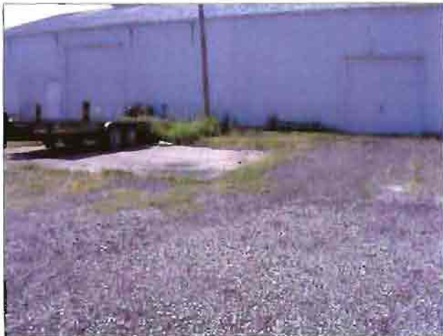
The parking lot at the Pets at Peace Crematory is deteriorated and has weeds growing out of it.
