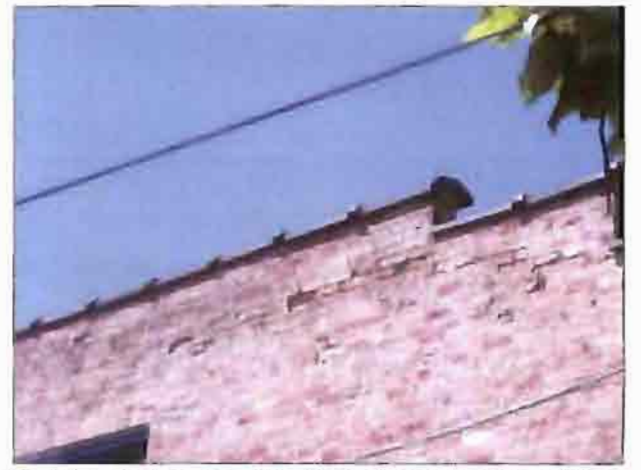
The bricks in the rear of the Hampshire Township building are crumbling.
