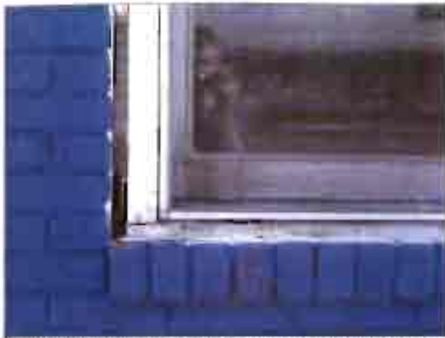
The window frame on the NAPA store show evidence of moisture damage.
