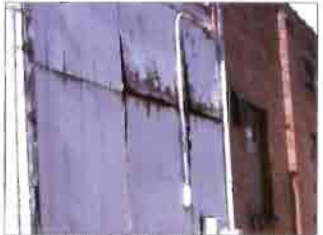
The wood panels on the rear of the Drey Miller meat building are rotting and separating from the structure.
