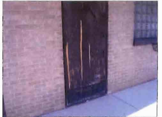
Front door of the Country Lanes Building is water damaged.
