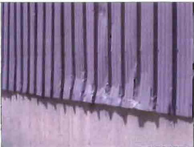
Large dents in industrial building south of Keyes Avenue.
