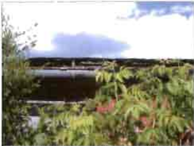
The vacant commercial building behind NAPA is missing sections of gutter. Note: overgrown weeds.
