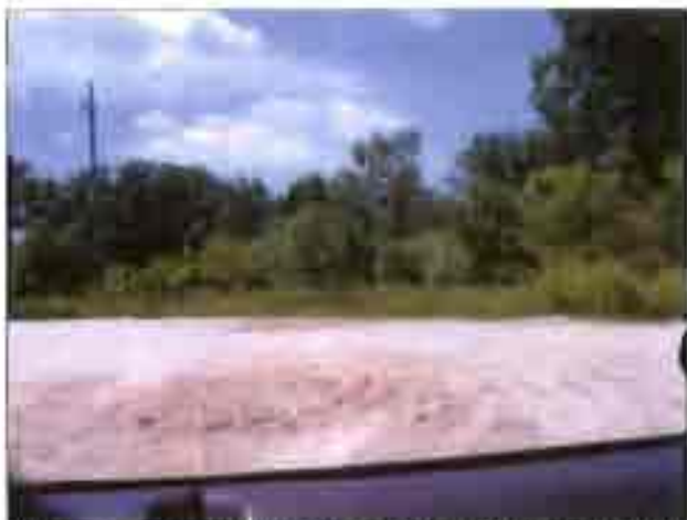
This unpaved parking lot north of Keyes Avenue has large depressions indicating poor drainage.
