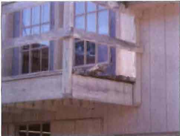
The porch on the front of the Fitness Center is unsafe. Note: rotting boards.
