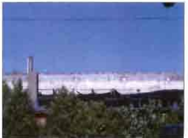
The rear of the roof on the vacant commercial building behind NAPA.
