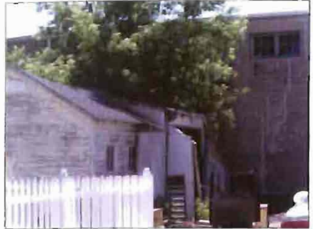
The Industrial building south of Keyes Avenue has severe step cracking.
