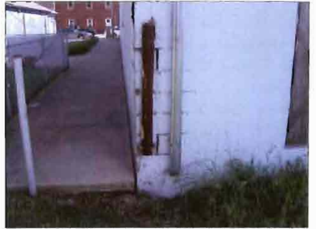
The rear of the Country Lanes building is in need of tuck pointing.
