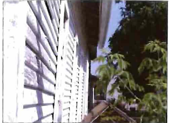
The exterior walls are leaning on the industrial building east of Center Street.
