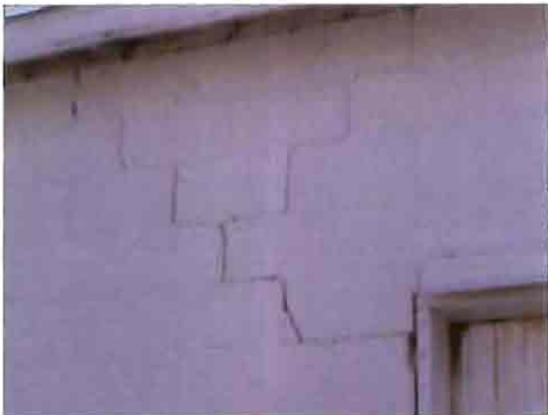
Step cracking in the masonry block wall on the industrial building east of Center Street.
