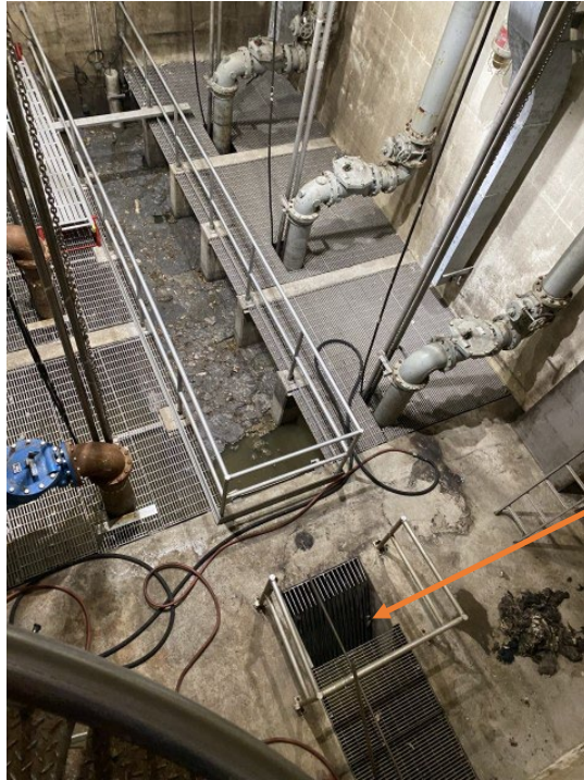
Influent Channel with Bar Rack
